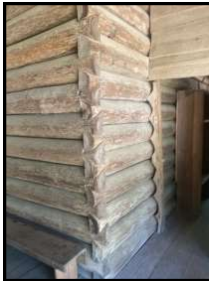
The corners of this log house were constructed using the half-dovetail notch technique which is self-locking and the most difficult type of notched corner to produce which reveals the remarkable carpentry skills of these pioneer farmers.
